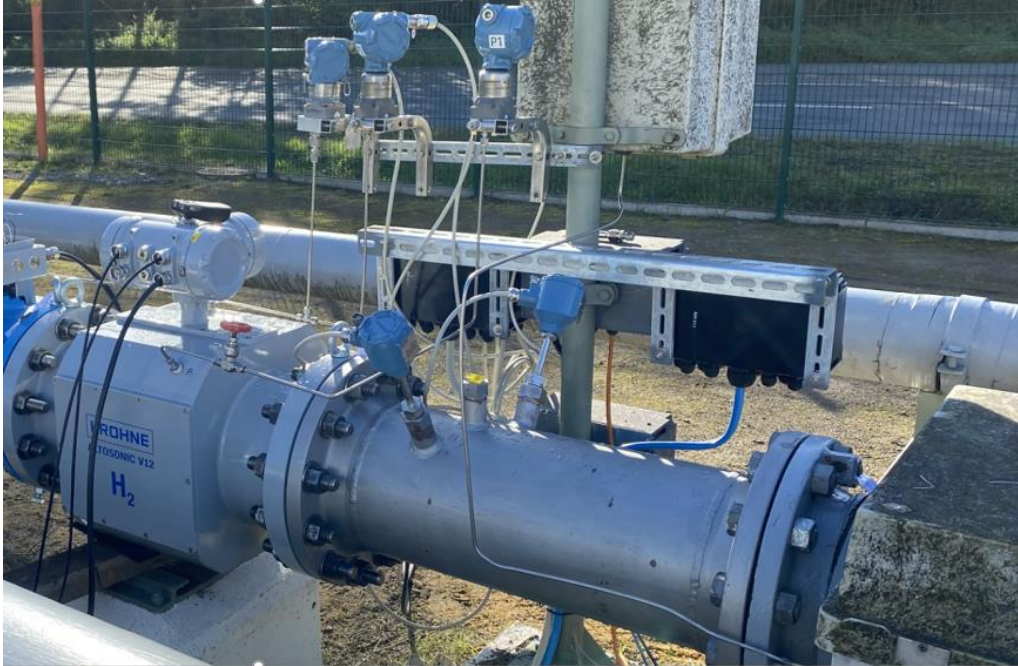
Figure 6: The 10" ALTOSONIC V12 (150#) ultrasonic custody transfer gas flowmeter installed on site.
