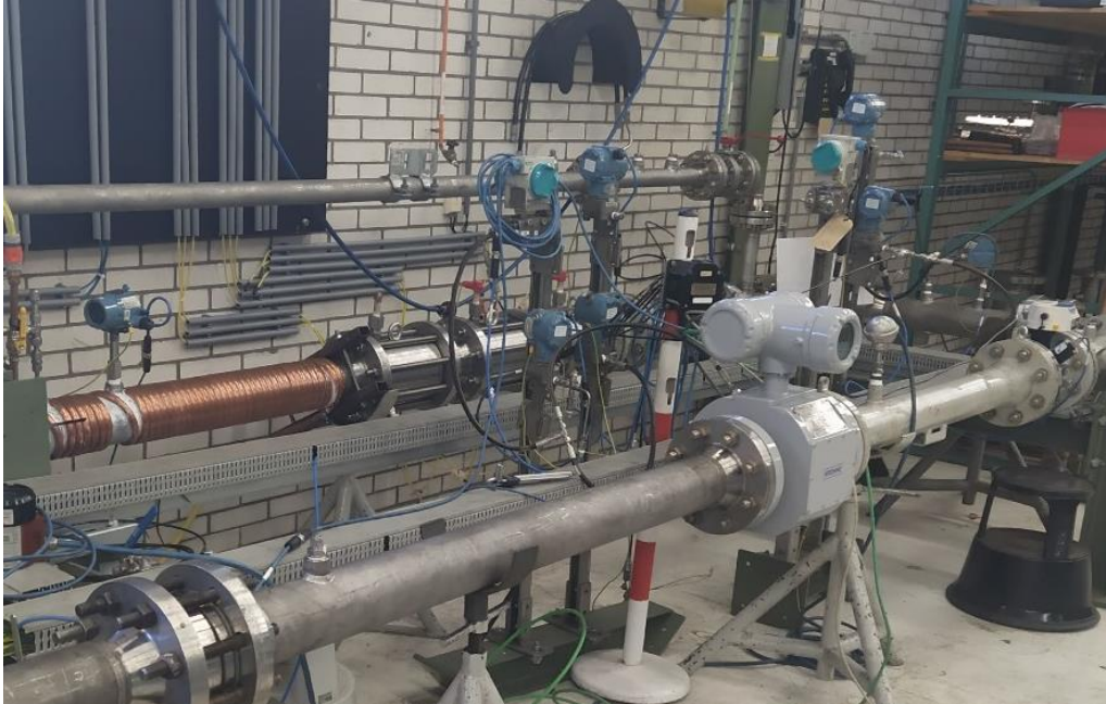
Figure 7: The 4" ALTOSONIC V12 ultrasonic custody transfer gas flowmeter installed at the DNV hydrogen test facility.
