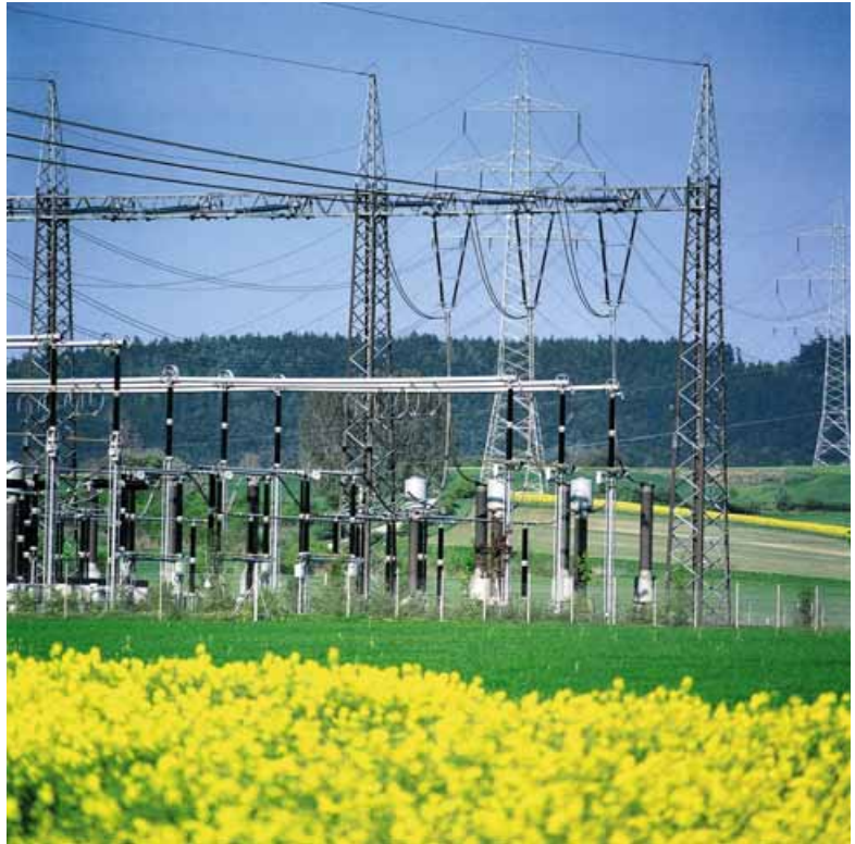
Fig. 26 400 kV outdoor switchgear
